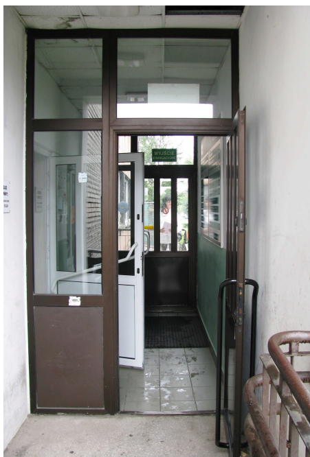
Picture 4. Entry door impeding wheelchair access
