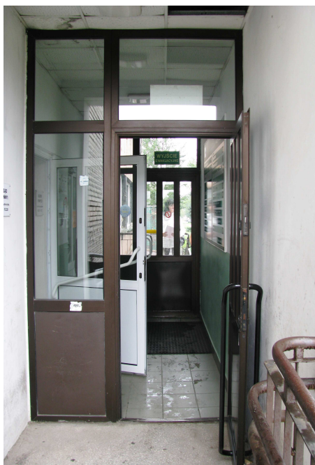
Picture 4. Entry door impeding wheelchair access
